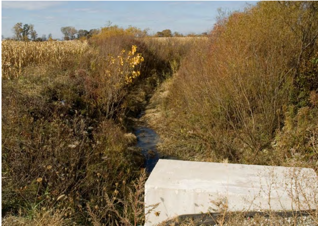
Plate 2: The LaChance Drain, west side of the intersection of Banwell Road and E.C Row Avenue.
