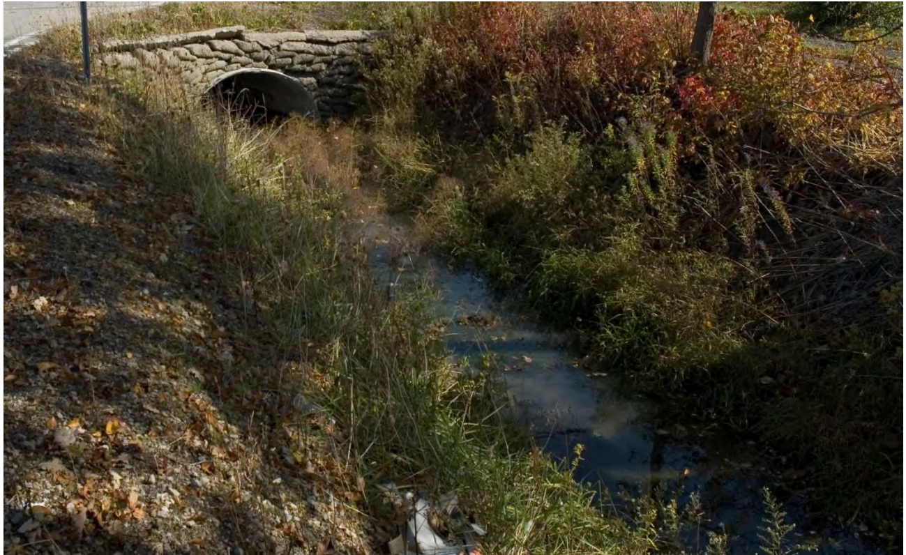
Plate 1: Gouin Drain culvert west side view of the intersection of Banwell Road and E.C Row Avenue.
