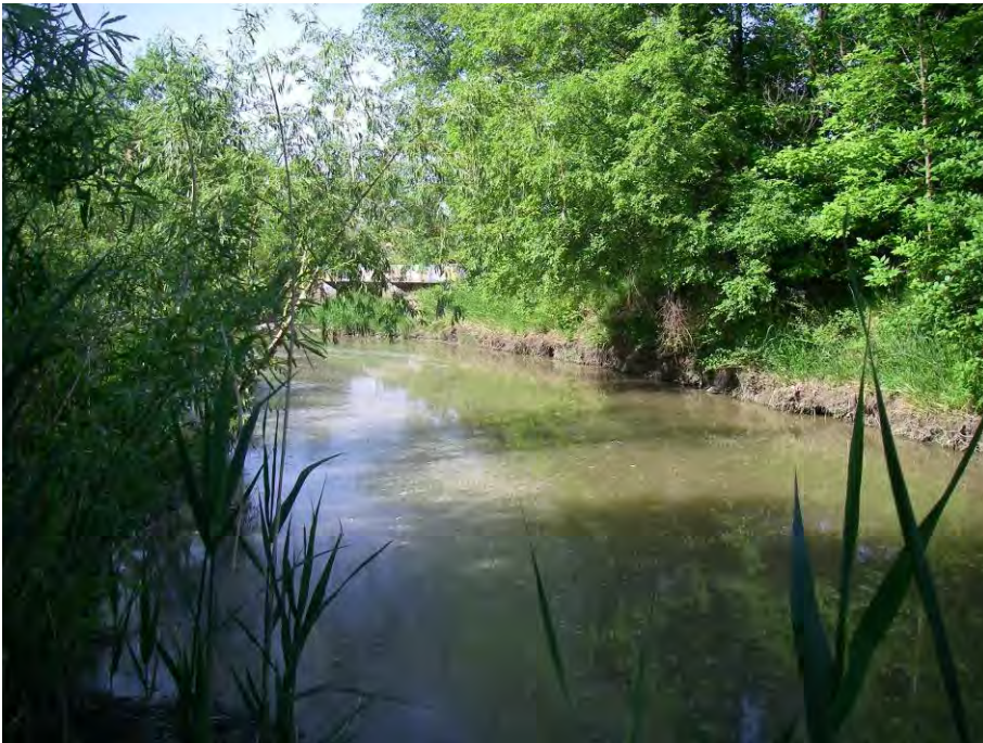
Little River Reach (LR-3) Looking at downstream end of reach at toe erosion of right bank
