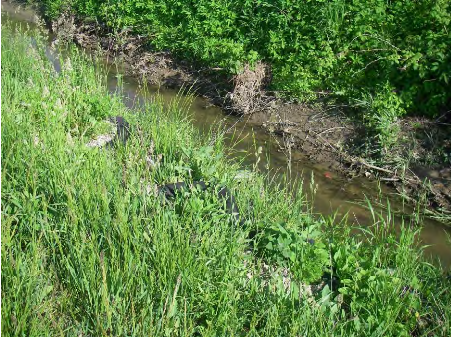
Sixth Concession (SCD-1) Looking downstream at right bank toe erosion
