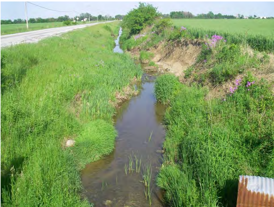
Baseline Road Drain (BRD-1) Looking downstream from end of reach at bank erosion
